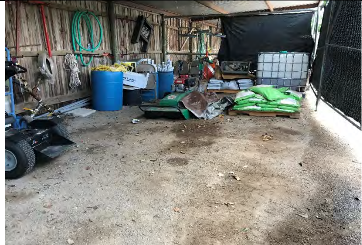
Photo 6: View of de minimis staining inside of equipment and materials storage shed on the east side of the Maintenance Barn area. Facing south.
