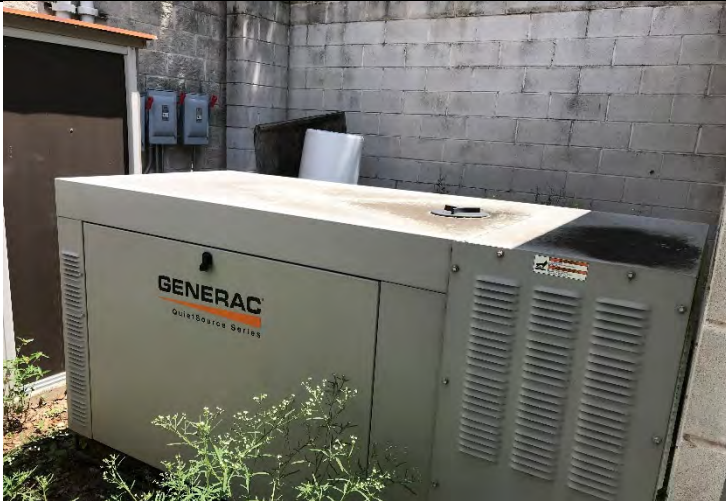
Photo 21: View of natural-gas fired emergency power generator on the south side of the Barton Creek Salamander hatchery building at the Nature Science Center. Facing east.
