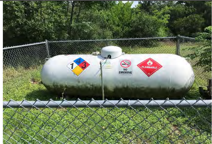
Photo 20: View of propane tank northeast of the Zilker Clubhouse. Facing north.
