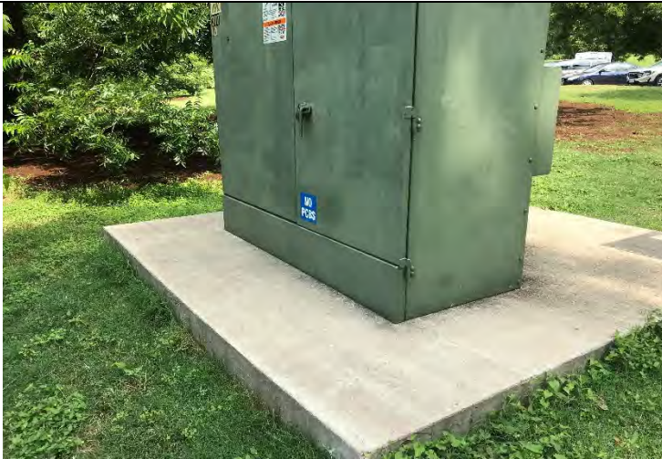
Photo 19: View of typical single pad-mounted transformer. This one is located in the southern portion of the Great Lawn. Photo facing southeast.
