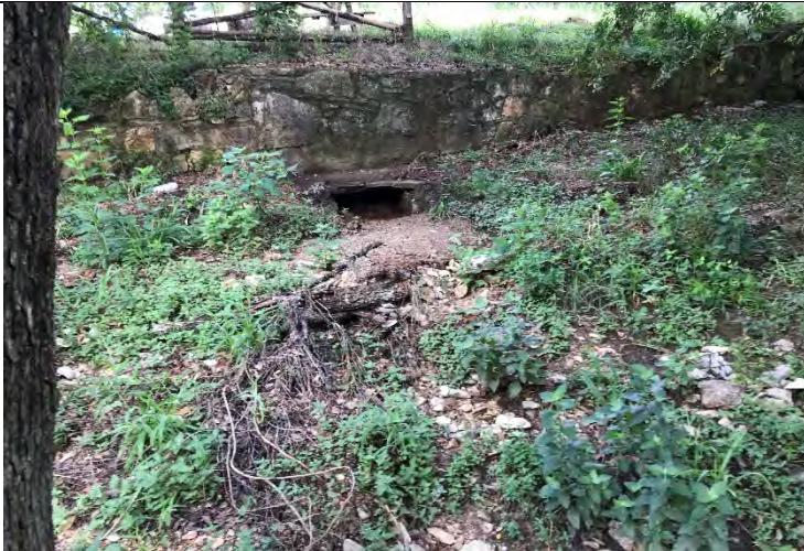
Photo 43: View of the outfall of the storm water conveyance on the east side of the Pistol Range. Facing west.
