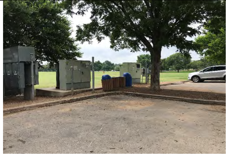
Photo 18: View of a typical pair of pad mounted transformers. These are located at the west side of the Great Lawn. Facing south.
