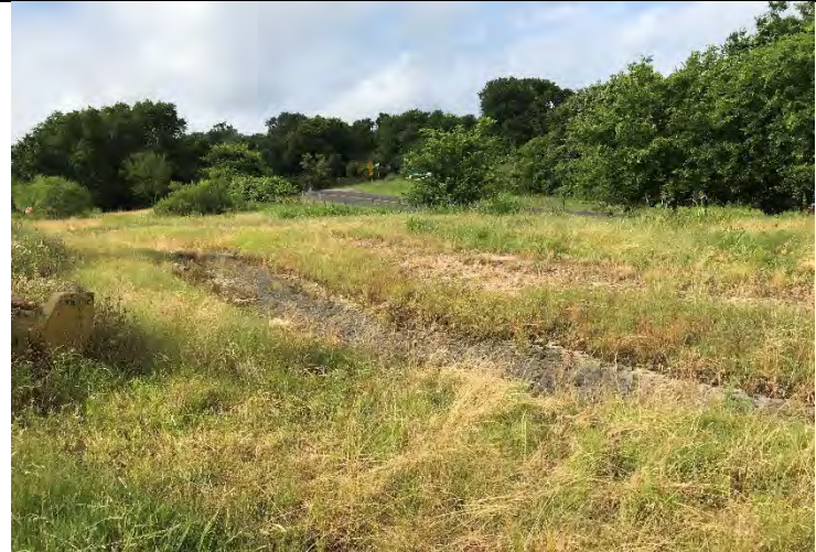
Photo 22: View of permeable interlocking concrete retaining blocks installed along Eanes Creek at the north end of the Bone Yard as part of erosion control improvements in this portion of the Butler Landfill. Facing west.
